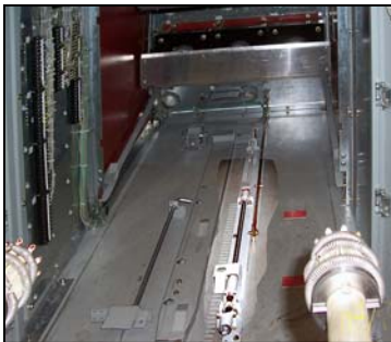
Fig. 3) Highlighted view of racking mechanism installed into a circuit breaker cell.
