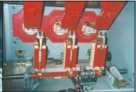
Grounding switch shown closed on breaker.
