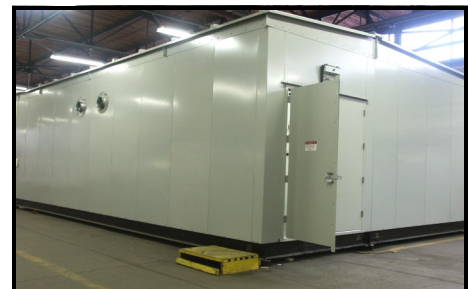
Typical Power and Control Center (PCC).
