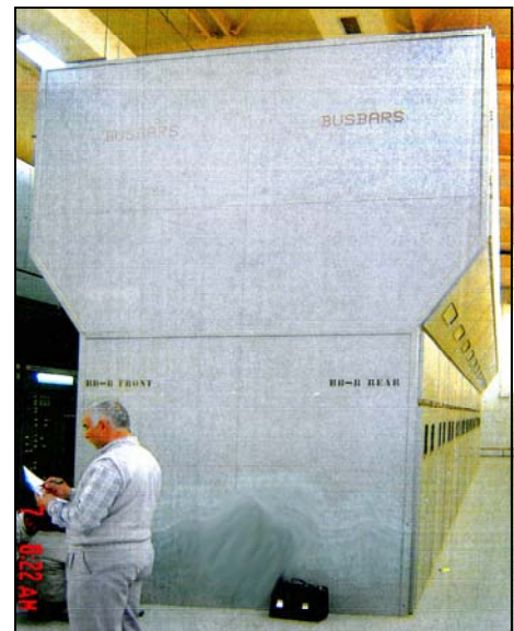
View of switchgear on site.
